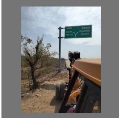
Overhead Cantilever Sign Board
